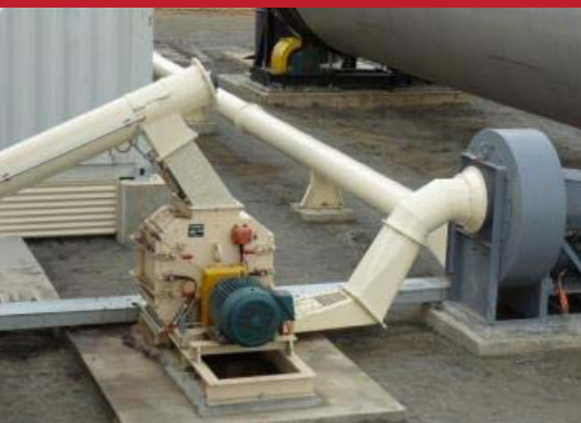
Hammer mill with pneumatic discharge fan and duct to horizontal cyclonic burner.
