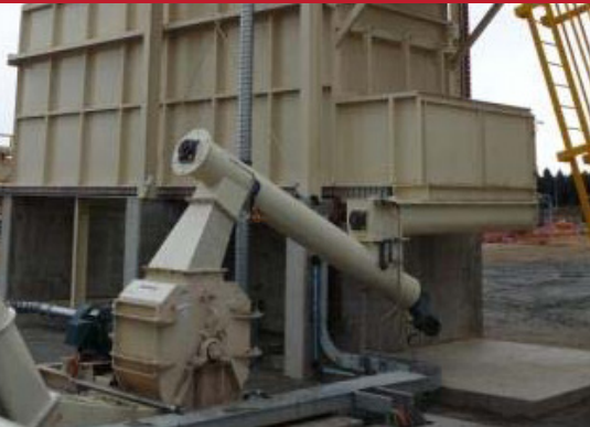
Storage bin with screw conveyor to hammer mill.
